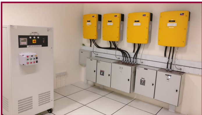
Close quarters: EPIC's transformer and inverter room
