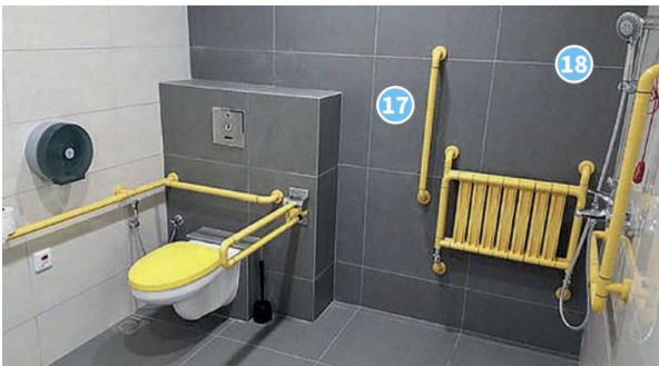
Figure 5: Examples of orientation cues for quick identification of the toilet. Good contrast of colours for fixtures and fittings.
