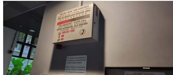
Figure 11. AAS device in void deck (Image credit: author)
