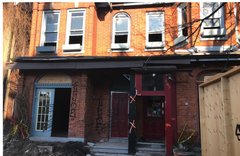
Figure 6.1 Derelict Heritage Housing in Toronto, Canada
