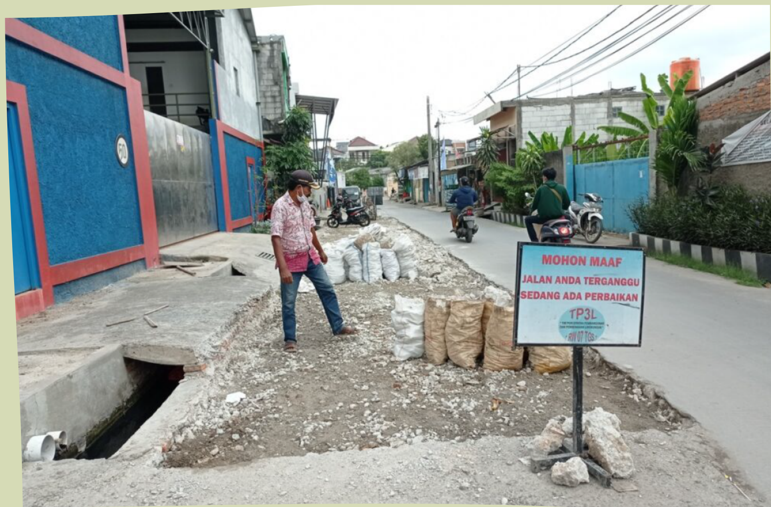
The revitalisation of the Perjuangan Road was financed through tolls collected from passing vehicles. Source: Kompas.com
